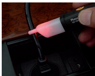
Incorrect phase sequence
